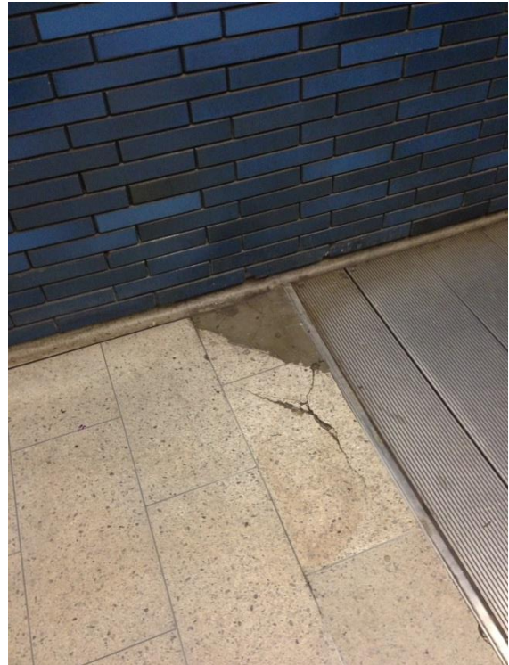
Floor in need of refurbishment
